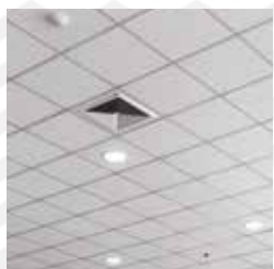
CEILING GRID FALSE CEILING
